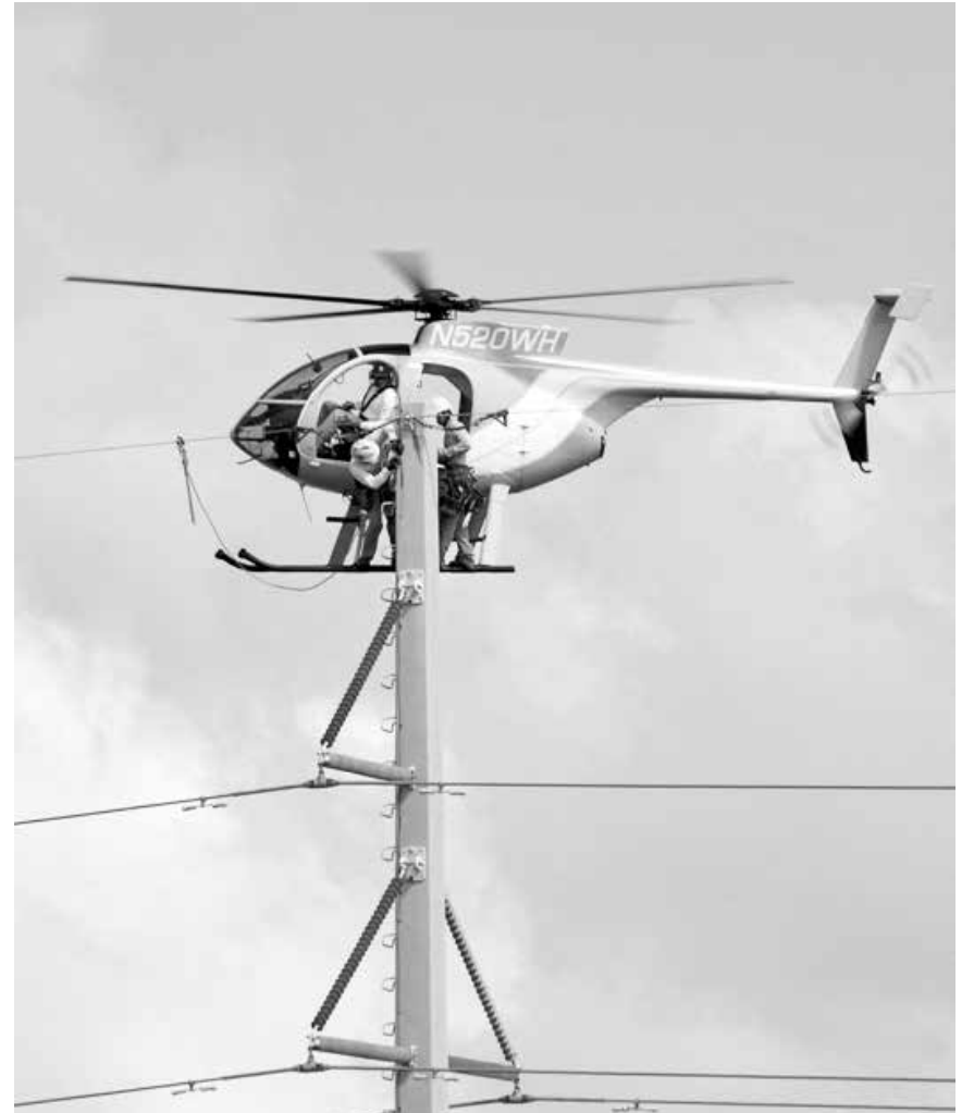
A helicopter completes inspections and repairs to the electrical tieline that powers the Florida Keys along U.S. 1. CONTRIBUTED
